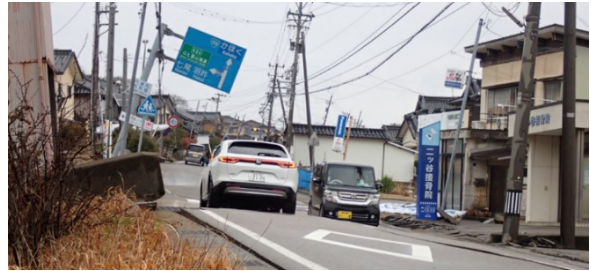
Figure 3, Cracks and Compressive Uplifts caused by lateral flow due to liquefaction (Uchinada-Town).
