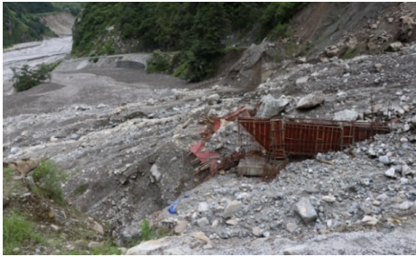
Figure 2, Under-construction Thaplyang bridge buried by a debris flow (piles sited in the active debris fan)
