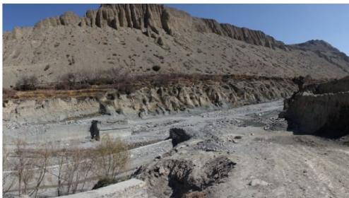
Figure 3, Destroyed Kagbeni bridge (collapse of the bridge deck, with only piles remnants).
