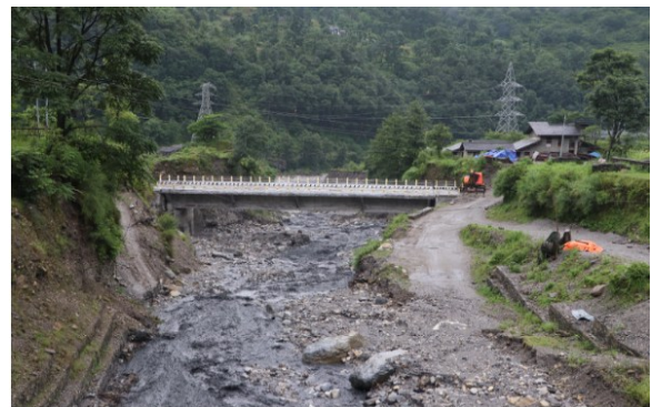
Figure 1, Bridge built in a downstream, narrower section of the Ghatte Khola, with piles in loose material.
