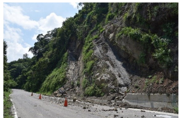
Figure 1, A collapse incident in 2022/08/29.
