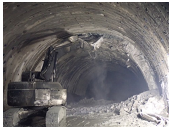
Figure 4 Re-excavation due to increased displacement.
