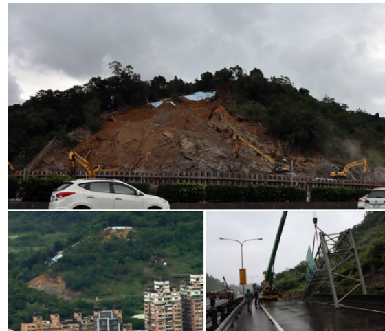
Figure 1, Dip-slope failure near national freeway no. 1 (Source: Geological survey and mining management agency).
