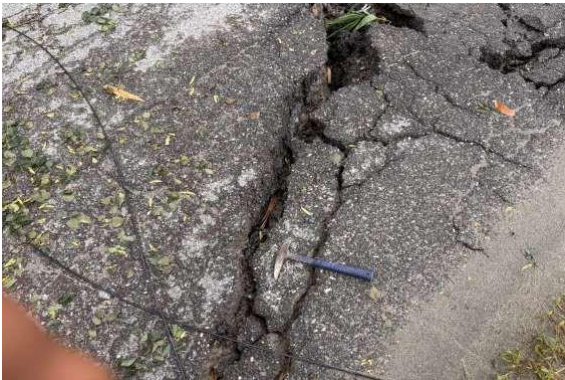
Figure 2, Tension crack in the road pavement at Krishna Bhir, showing lateral displacement of the road surface.
