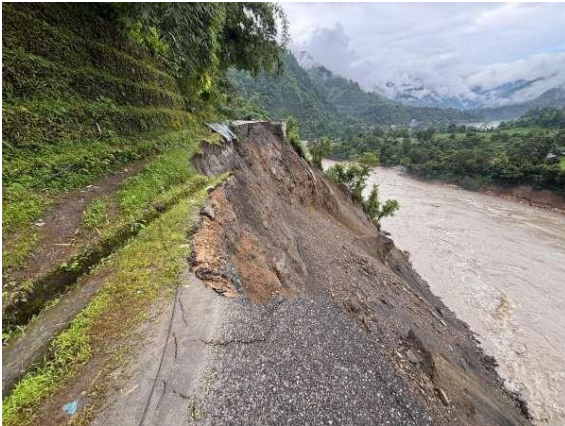
Figure 1, Toe erosion and collapse of the Prithvi Highway above the Trishuli River at Krishna Bhir.
