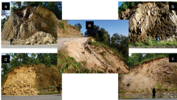
Figure 1, Representative slope conditions along the selected road section; a) Rockfall at Jitpur Bhanjyan, b) Joint sets at Taplakhar, c) Slope condition at Shikhar Kateri, d) Rock fall at Shikhar Kateri and e) Down slope failure at Bar Bhanjyan.
