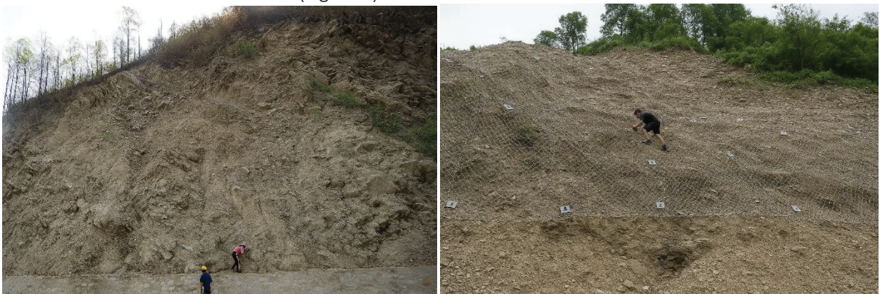
Figure 3, Field photographs of rock-cut slopes
